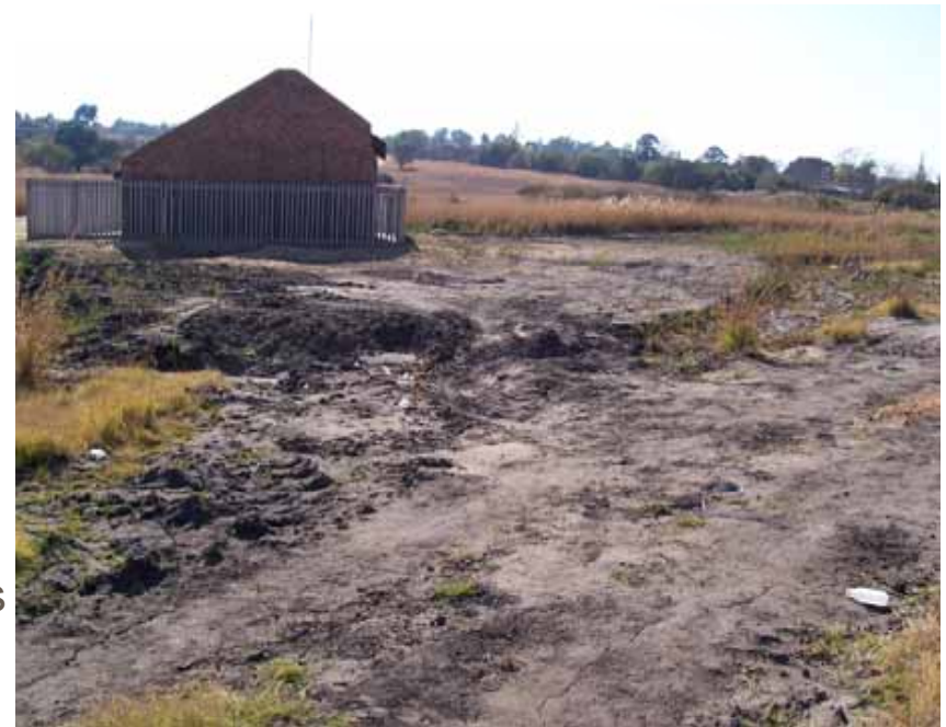
Sewer pump station in a wetland, Blue Hills
